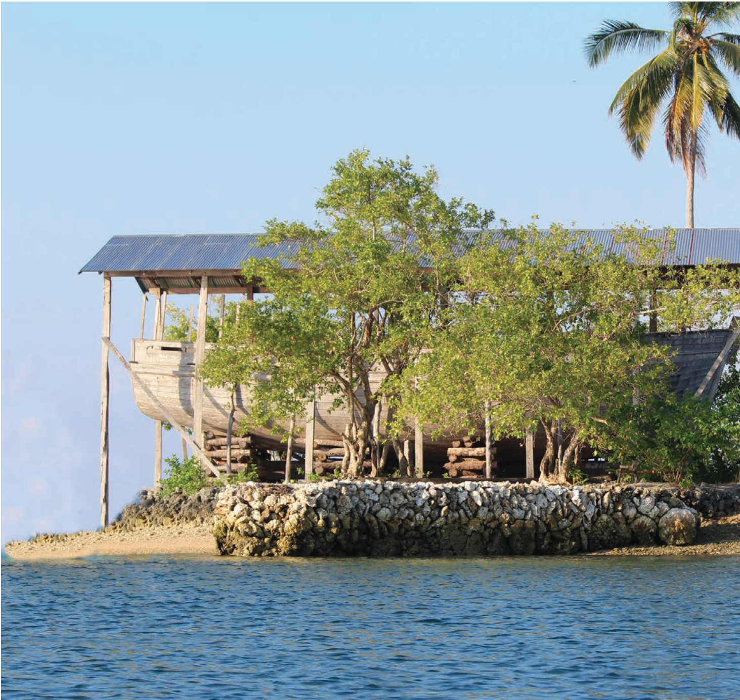
A timber boat under construction in one of the many artificial islands that dot Langa Langa Lagoon.
